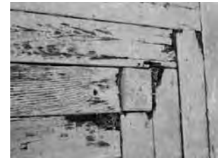
Close up of the condition of the old deck.
