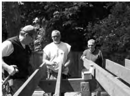
The construction team worked like a pro crew and created a deck that was not only beautiful, but structurally sound for this busy family.
