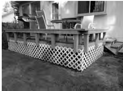
Rot and mildew were just two of the problems the old deck posed the homeowners.
